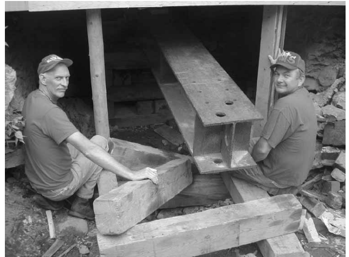
Historical Society member Ed Fowler confers with contractor Lester before the house is raised.
