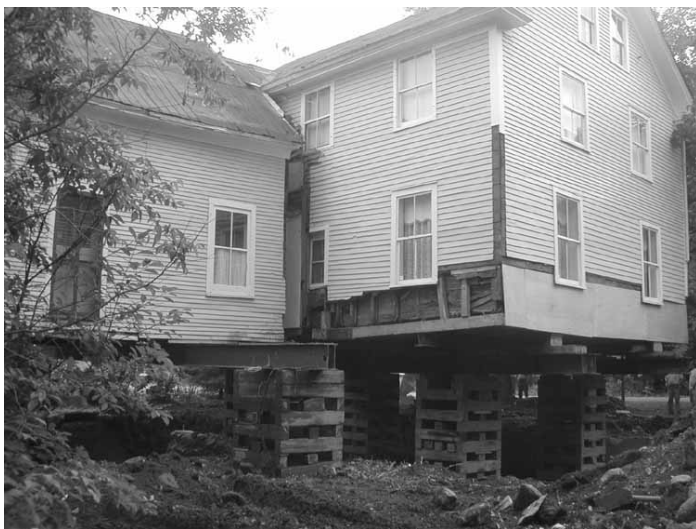
The museum is finally lifted off what is left of the crumbling former foundation.
