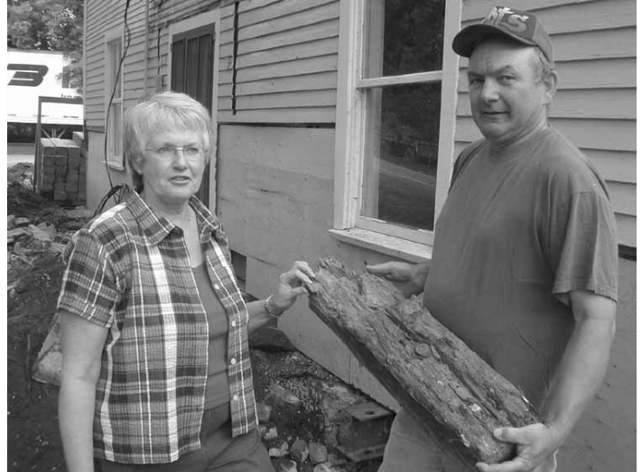
Contractor Earl Lester shows society member Judy Laberee one piece of a rotten beam pulled out from the bottom of the house.
